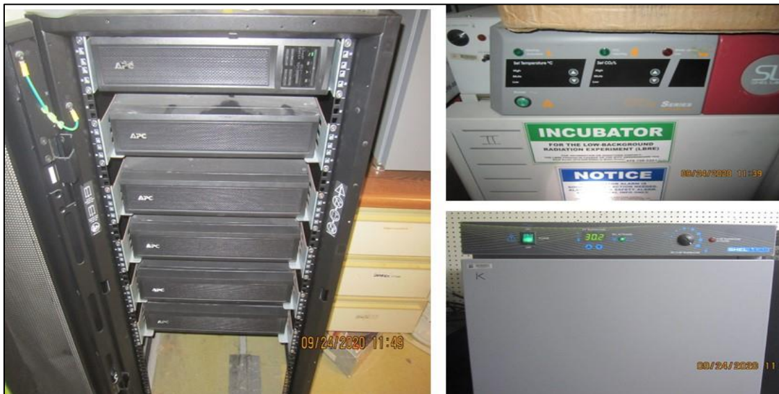
Figure 10.1. Left photo: Uninterrupted Power Supply (UPS ) installed in the LBRE lab underground at WIPP in Oct. 2019. Top right shows the old incubator, bottom right the new Peltier incubator
