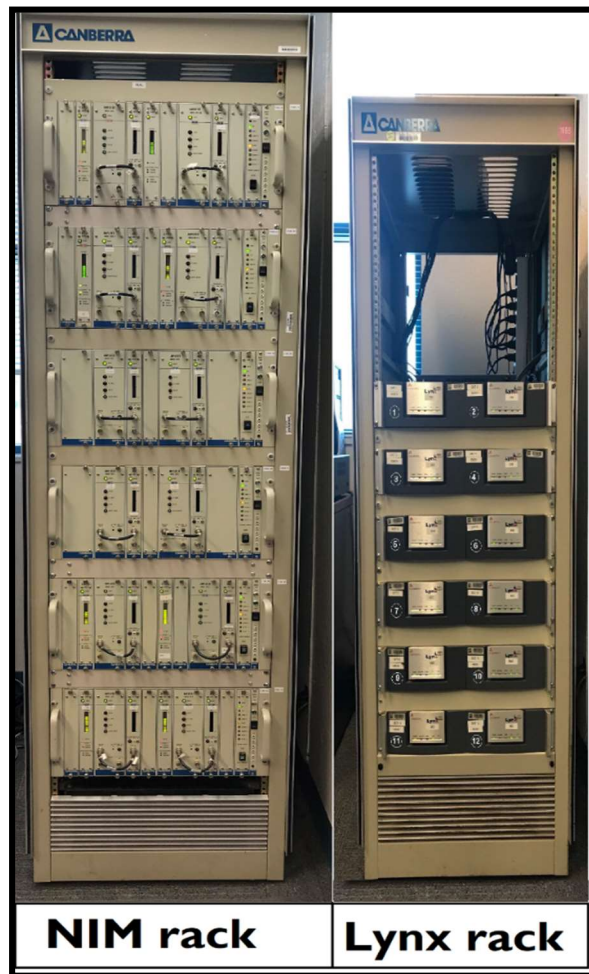
Figure 9.2. NIM and Lynx racks with electronic units
